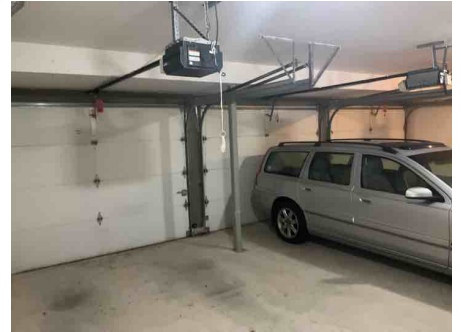
Unprotected garage doors
